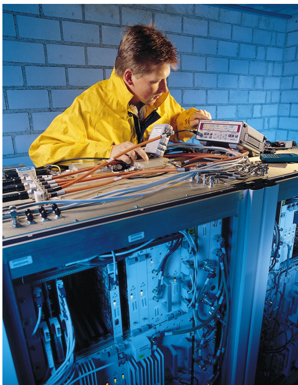
FIG 5 Power Reflection Meter NRT and 4-GHz Directional Power Sensor NRT-Z44: competent tools for on-site applications, here during installation of mobile-radio base station Photo 42 667/1
