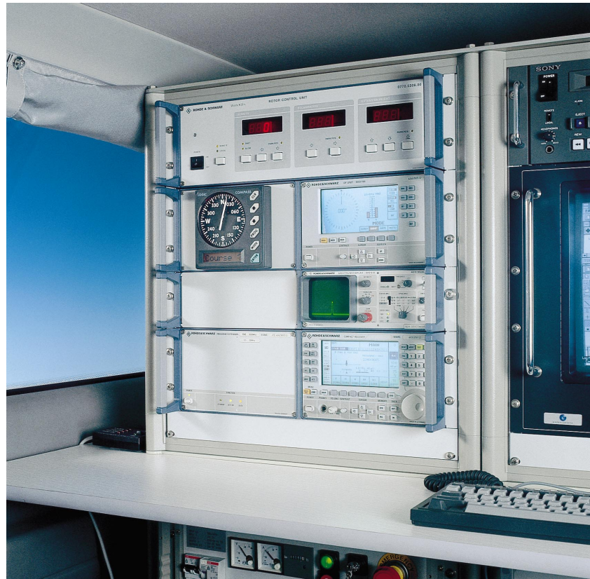
FIG 3 Compact radiomonitoring and radiolocation system in mobile DF unit: VHF-UHF Receiver ESMC with Frequency Extension ESMC-FE, Panoramic Display EPZ513, VHF-UHF Direction Finder DDF190, compass and antenna controller Photo 42 611/9
